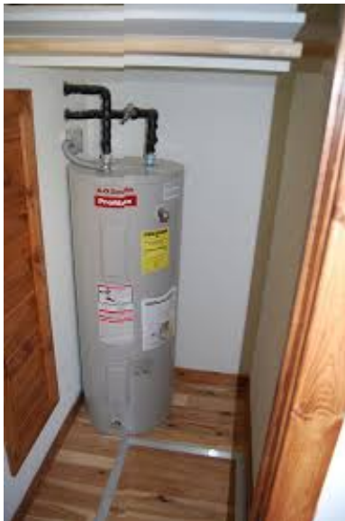
Typical Water Heater
