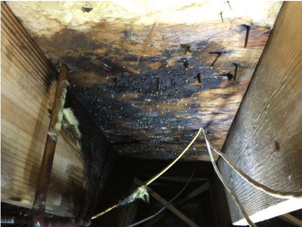
Because of moisture, MOLD can easily grow and spread in crawl spaces.
